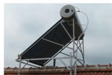
storage on the top and collector panel on the bottom.
